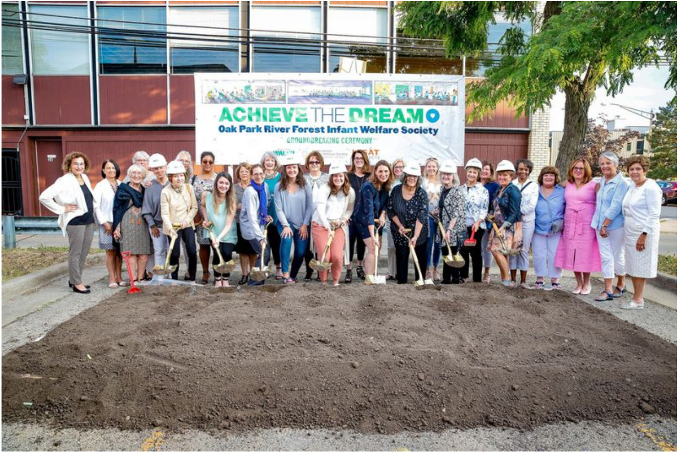
Supporters of the Oak Park River Forest Infant Welfare Society participated in a "groundbreaking" ceremony for the nonprofit's new 10,000-square-foot building on Madison in Oak Park. - Original Credit: OPRF Infant Welfare Society (OPRF Infant Welfare Society / HANDOUT)
